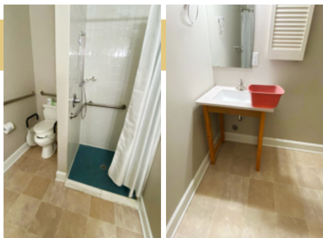
These photos were taken at a reputable senior living facility. Note how water could easily pool in the shower, increasing the risk of a fall; and the lack of grab bars and support around the sink at right.
